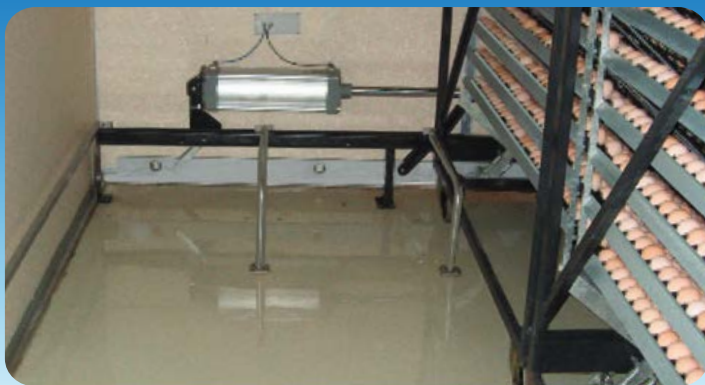
Fig 1: Standing water on the floor of a single stage setter at the end of the sealed period.
